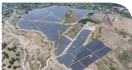
105MWp BINALONAN SOLAR POWER PLANT
