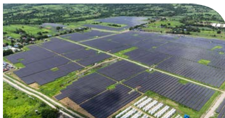
177MWP SOLAR BOLBOK 1 & 2
