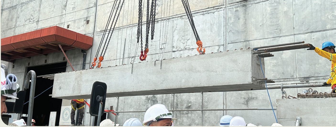
Megawide Construction Engineering team and Sumitomo team successfully conducted the SQRIM mock-up.
