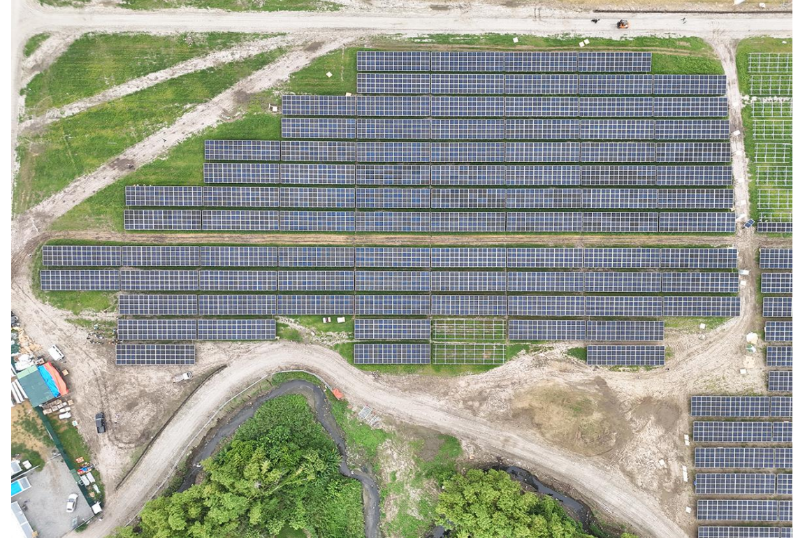
ARAYAT SOLAR POWER PLANT
