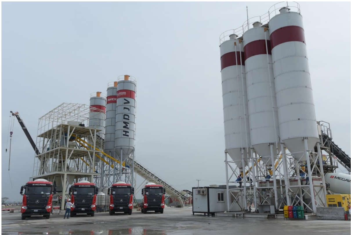
CAPTION: The Megawide mobile concrete batching plant in Apalit, Pampanga, built to supply concrete for the Malolos-Clark Railway Project Package 1
